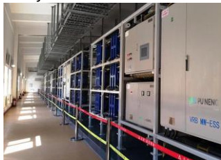
8 MWh VRB in Zhangbei, China
